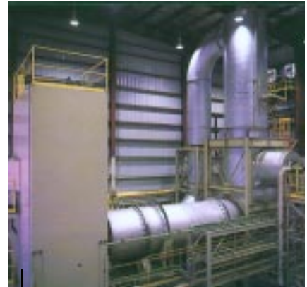
Industrial Waste Rotary Incineration System
