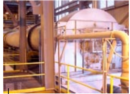
Direct-Fired Rotary Kiln for Calcining Bauxite
