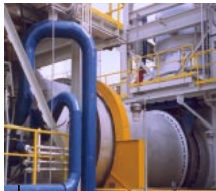
Rotary Incinerator for Hazardous Wastes
