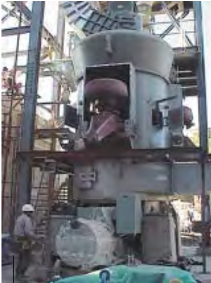
HP Bowl Mill Installation
